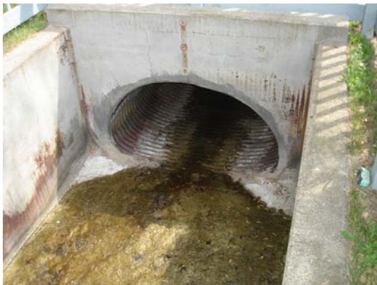
Name: DSC00130 Date Modified: 7/26/2006 11:37:08 AM Date: 7/26/2006 11:37:08 AM Description: Upstream face of pipe under driveway
