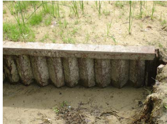
Name: DSC00138 Date Modified: 7/26/2006 11:39:20 AM Date: 7/26/2006 11:39:20 AM Description: Rusted sheet pile of control structure
