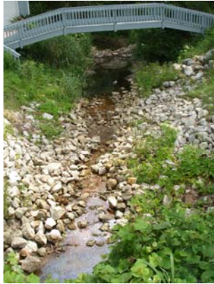
Name: DSC00128 Date Modified: 7/27/2006 8:55:00 AM Date: 7/27/2006 8:54:58 AM Description: Looking downstream of control structure
