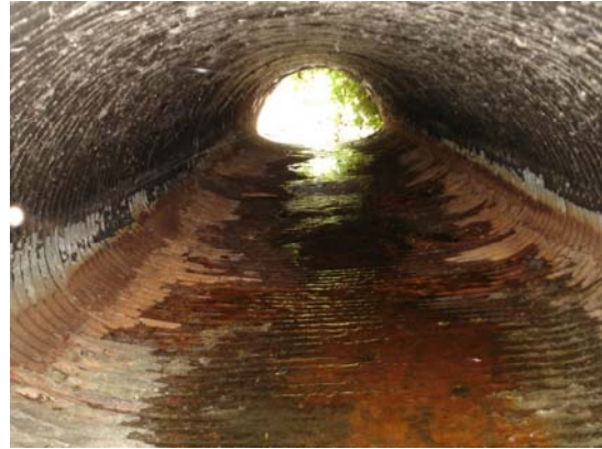
Name: DSC00142 Date Modified: 7/26/2006 11:40:26 AM Date: 7/26/2006 11:40:26 AM Description: Rusted CMP pipe under driveway
