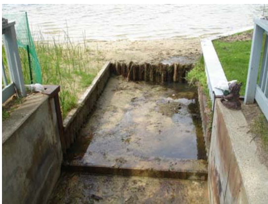
Name: DSC00132 Date Modified: 7/26/2006 11:37:54 AM Date: 7/26/2006 11:37:54 AM Description: Looking upstream at control structure
