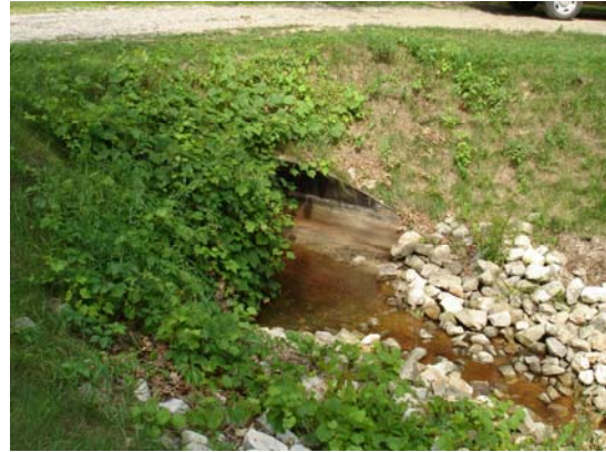
Name: DSC00129 Date Modified: 7/26/2006 11:36:22 AM Date: 7/26/2006 11:36:22 AM Description: Downstream face of pipe under driveway
